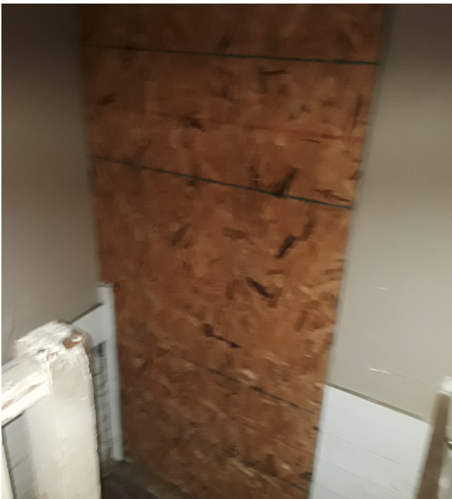
Base Stair 13, Side C - Boarded shut
